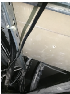
Example of large cable penetrations in electrical risers - no fire stopping
