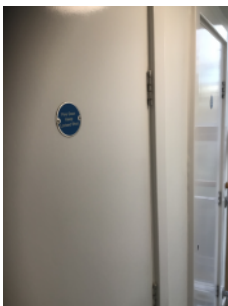
“Fire door keep locked” signage on timber riser doors.
