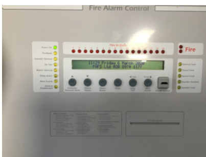
Fire alarm control panel
