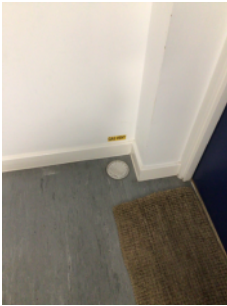
Gas vent within corridors
