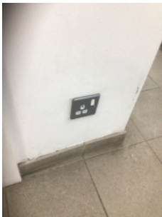
Electrical sockets in common areas throughout the building
