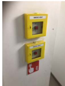
Smoke ventilation manual actuators
