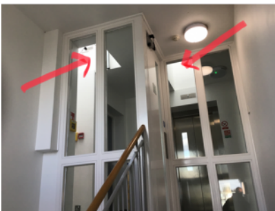
6th floor partition viewed from staircase showing position of AOVs
