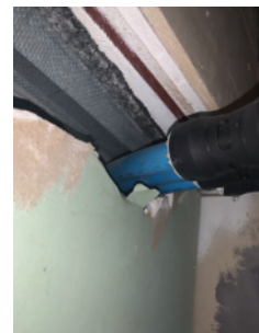
Example of large pipe penetrations in gas/water risers - no fire stopping
