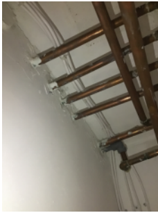
Example of fire stopping within riser cupboards.
