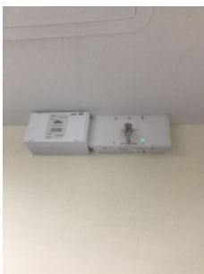
Wireless devices installed in each flat.
