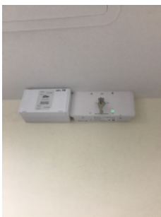
Wireless devices installed in each flat.
