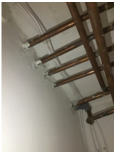
Example of fire stopping within riser cupboards.
