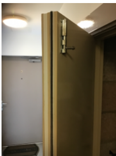
FD60S doors installed in risers
