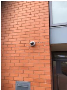
External CCTV Camera
