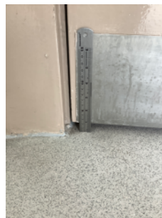
Lobby door threshold gap of 20mm
