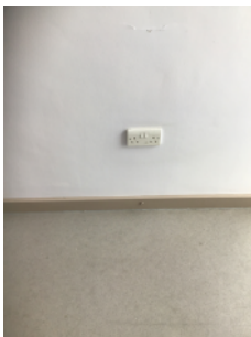
Electrical sockets in common parts
