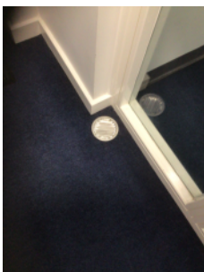
Gas vents in common corridors
