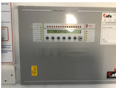
Fire alarm control panel
