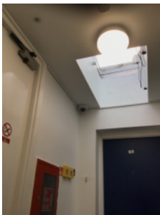
AOV located in 6th floor lobby.
