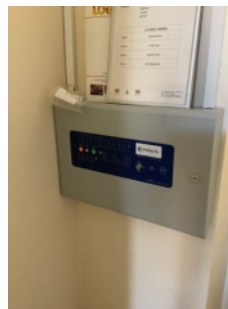
Panel in "healthy" condition.
