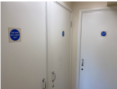
Fire door keep locked shut signage on electrical cupboard doors.
