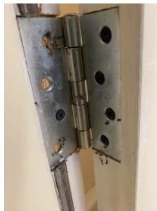
Screws missing from hinges on electrical cupboard door.
