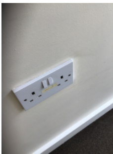
Electrical sockets provided in staircase
