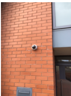
External CCTV Camera
