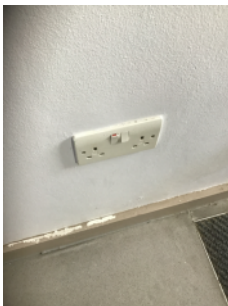
Electrical sockets in common parts
