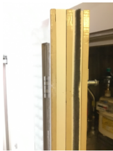
FD60S doors installed in risers
