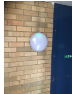
Maintained EL provided in the staircase.
