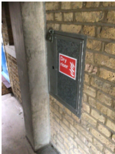
Dry riser outlets provided on each floor.
