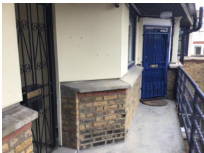
Security gates across flat entrance doors.
