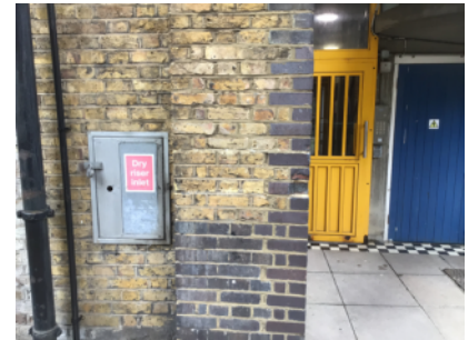
Dry riser inlet provided outside main entrance door.
