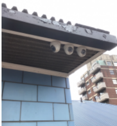
CCTV cameras are provided.
