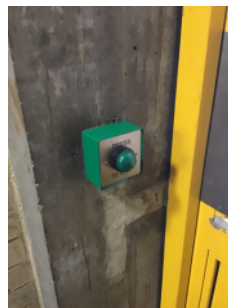
Exit device provided on main entrance door.
