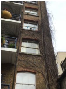
Dry/dead vegetation on the side of the building should be removed
