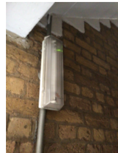
Non-maintained emergency lighting in the staircase
