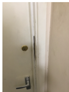
Damaged door frame
