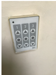
Vent controls that do not appear to work
