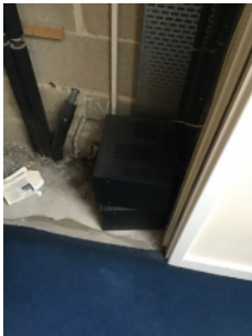
Storage in riser cupboard on the third floor.
