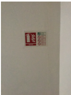
Old extinguisher signage
