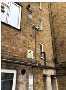
External CCTV cameras
