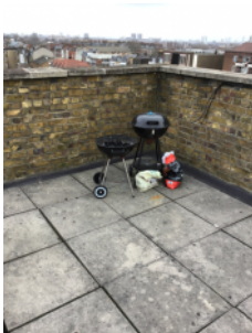
Barbecue located on building roof.
