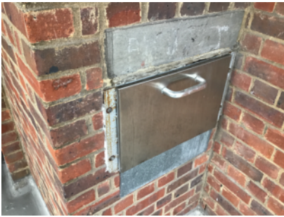
Well fitted, appropriate standard, rubbish chute hatch.
