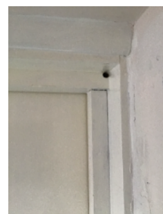
Small hole in door frame.
