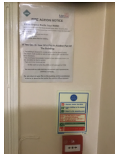
Conflicting Fire Action Notices in No.20A
