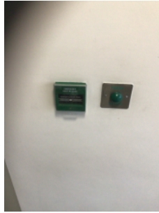
Electromagnetic door release with emergency door release, staircase doors.
