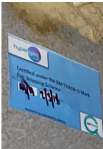
Evidence of certification fire stopping within riser cupboards.
