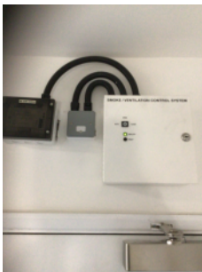
Smoke ventilation control system and fire alarm interface in staircase
