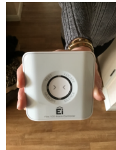
Remote wireless fire alarm controller installed in each flat
