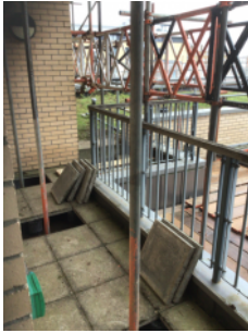
Hazardous route to and from roof garden created by the scaffold currently i
