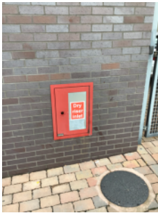
Dry riser inlet
