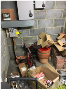
Combustible waste in electrical room
