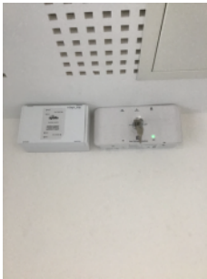
New fire alarm interface key in the off position.
