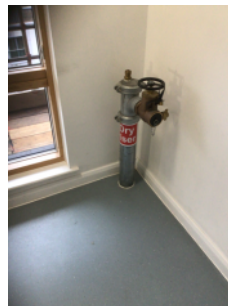
Dry riser outlet on staircase landings.
