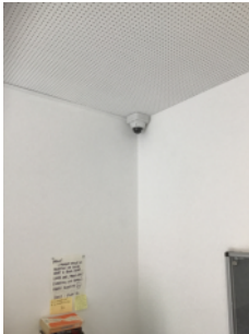
CCTV cameras are installed internally and externally.
