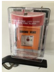
Incorrect signage on AOV control
