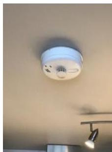
Interlinked kitchen heat alarm, flat 28
