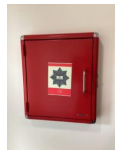
Premises information box
