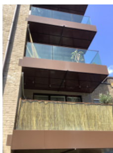
Combustibles on private balconies
