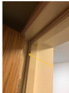
Flat 28- possibly surface mounted smoke seal
