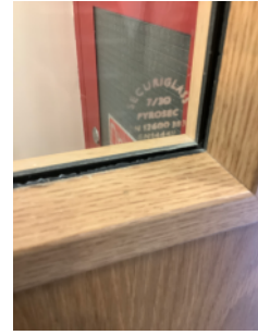
Acid etching on FR Glazing installed in staircase doors.
