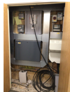
Main electrical intake and landlord's distribution board
