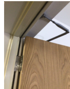
Self closer with intumescent strips and seals, staircase lobby
