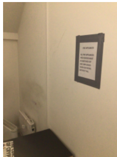
Fire safety notice for fire wardens attention
