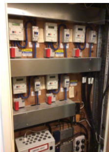
Electric meters in riser cupboard
