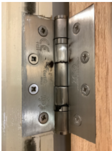
BS EN1935 fire rated door hinges in staircase doors
