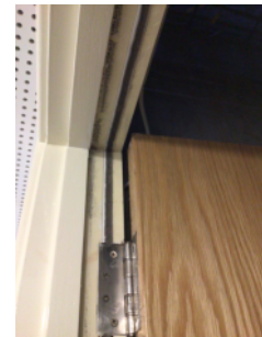
Intumescent strips and cold smoke seals installed on smoke shaft doors
