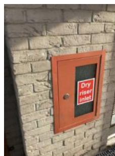
Dry riser inlet
