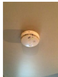
Interlinked hallway smoke alarm, flat 28
