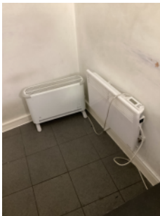
Heaters in stairwell
