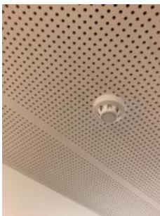
AOV operating smoke detector
