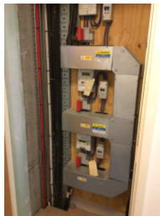
Electrical meters within riser cupboard
