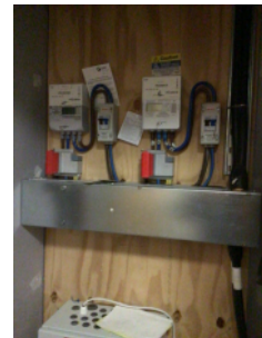
Electric meters in riser cupboard
