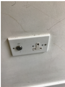
Electrical sockets with isolator lock in common areas
