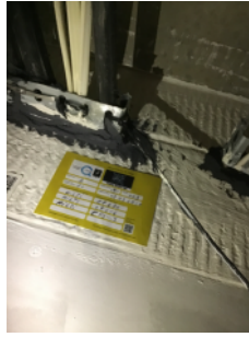
Evidence of fire stopping in riser cupboards, carried out in March 2020
