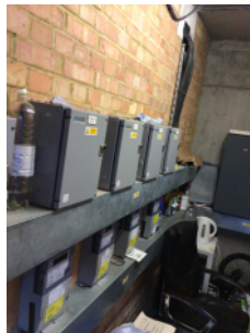
Electrical intake room
