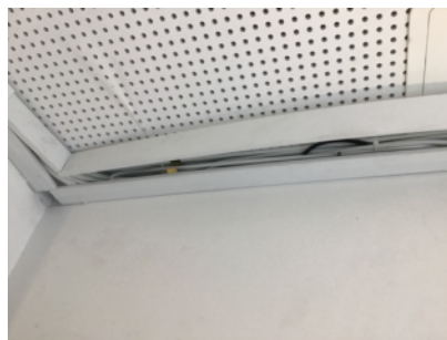
Showing cables within plastic ducting affixed to the ceiling in common area
