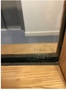
Acid etching on FR Glazing installed in staircase doors.
