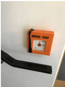
Smoke Vent controls held shut with tape
