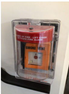
Incorrect signage on AOV control
