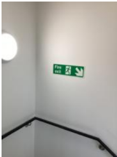
Escape route signage
