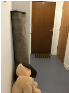
Combustible items outside of flat 9
