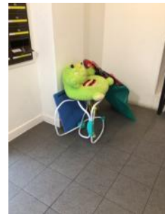
Combustible items in main entrance
