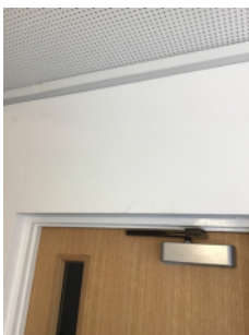
Cable runs in plastic trunking above staircase door.
