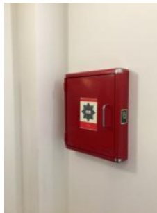
Premises information box
