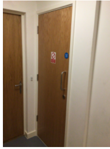
Electrical riser cupboard door
