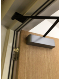
Self closer with intumescent strips and seals, staircase lobby door
