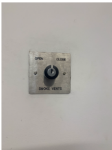
Manual smoke vent controls
