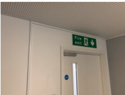
Example of PVCu cable conduit over staircase door.
