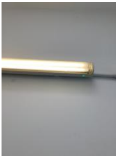
Stairwell emergency lighting
