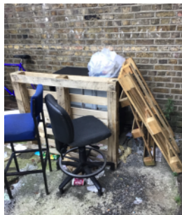
Combustible waste in rear yard.
