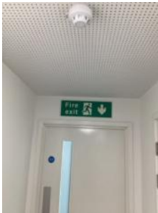
Escape route signage
