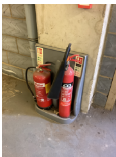
Plant room extinguishers
