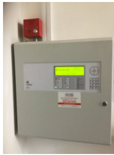
Fire alarm panel in entrance lobby.
