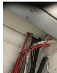
Example of poor fire stopping in some electrical risers
