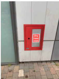
Dry Rising Main inlet
