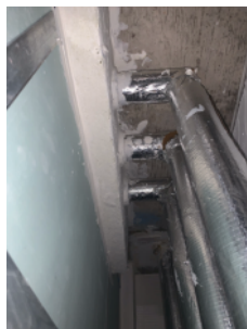
Example of good fire stopping in some areas
