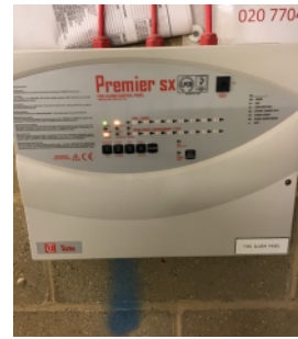
Version 4 - fault light on fire alarm panel in plant room
