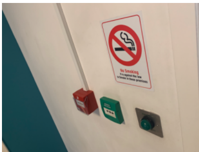
Manual call points located at each floor exit
