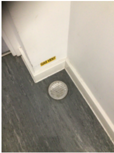
Gas vent in common corridors.
