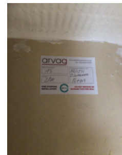
Fire stopping certification within riser cupboards
