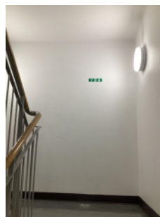
Inadequate escape route signage
