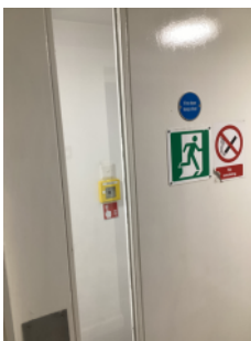
Escape route signage
