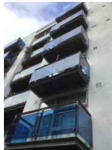
Configuration and construction of private balconies on the front elevation of the building
