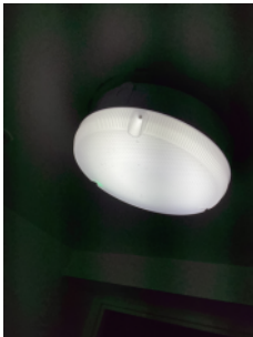
Emergency lighting unit
