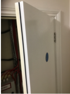
FD30S fire doors installed in riser cupboards
