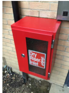
Dry riser inlet adjacent main entrance door.
