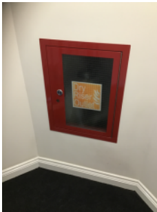
Dry Riser outlet in staircase
