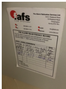
Evidence of Smoke Ventilation System test - 25.02.2020
