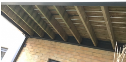
Photo showing the timber deck and joist construction of private balconies External wall details
