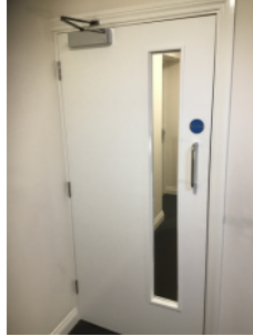
FD30S Self-closing doors provided in the staircase
