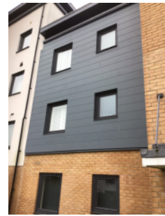
External wall system fitted to 1st and 2nd floors of rear elevation
