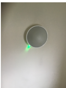
Maintained EL provided in the staircase
