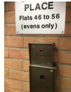
Entrance door override, tested and found to be working satisfactorily
