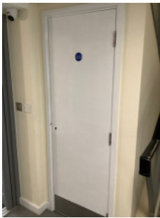
It was not possible to access this door due to a non-standard lock fitted
