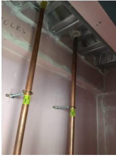
Example of compartmentation and fire stopping within gas riser cupboards.
