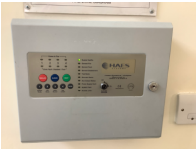
Control panel, showing “Healthy” condition
