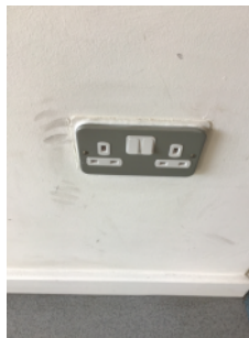
Electrical sockets in common areas.
