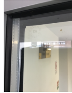
Acid etching on staircase (balcony access) door glazing.
