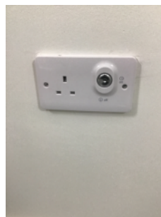
Electrical sockets in common areas, with security lock
