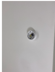
Missing smoke detector at head of staircase on the third floor.
