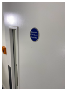
“Automatic fire door keep clear” signage provided on Staircase doors
