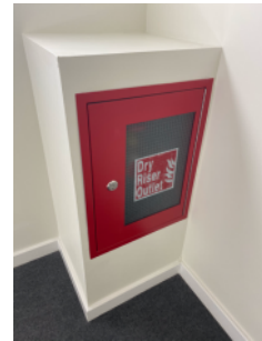
Dry riser outlets located within the staircase
