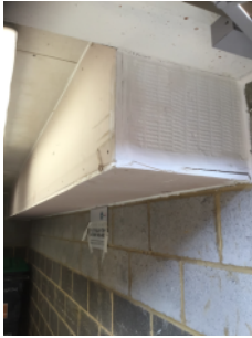
Fire stopping within the bin store
