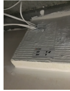
Certification label on fire stopping, meter cupboard, 2nd floor.
