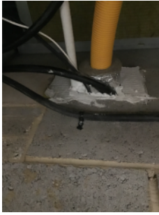
Example of acceptable fire stopping within electrical cupboard.
