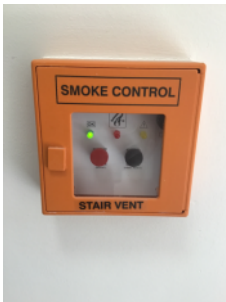
Smoke control override, showing status "ok"
