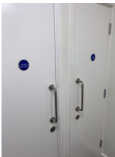
“Fire door keep locked” signage provided on riser cupboard doors
