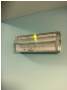
Non maintained emergency lighting unit in staircase
