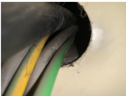
Penetrations from meter cupboards (not FR) on staircases into risers.
