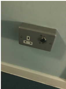
Electrical sockets in common areas.
