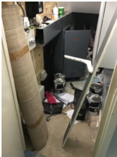
Paint and other combustible items in the electrical cupboard.
