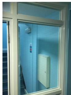
Georgian wired glazing
