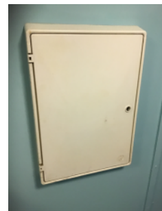
UPVC electrical meter cupboards in staircases.
