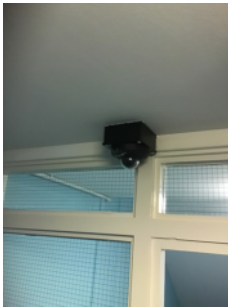
Internal CCTV camera
