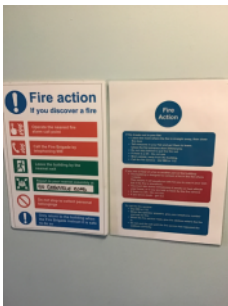
Conflicting fire Action Notices in place.
