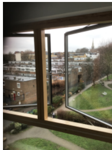
Window AOV on the 4th floor
