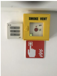
Smoke ventilation control
