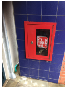
Dry riser inlet located directly outside main entrance door.
