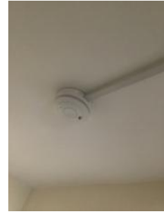
Flat 4 smoke alarm
