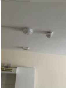
Heat alarm and detector flat 4 kitchen.
