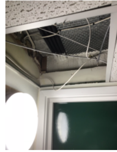
Evidence of fire stopping above suspended ceiling
