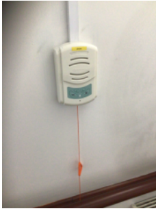
Telecare call-points are provided in common areas and within flats.
