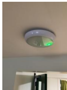
Emergency lighting unit
