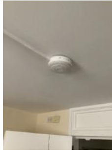
Smoke alarm flat 4
