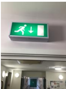
Maintained escape route signage
