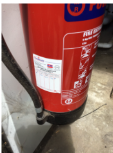
Dry powder extinguisher in boiler requires testing
