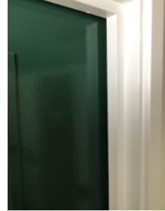
Corridor door not closing fully
