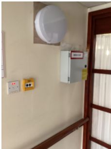
Smoke vent control and manual control
