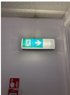
Maintained escape route signage
