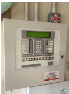
Fire alarm panel
