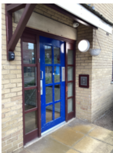
Secure front entrance door
