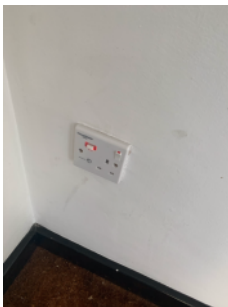
Electrical sockets in the staircase.
