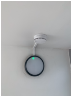
BS5839-6 Fire Alarm at the head of the staircase
