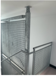
Structural staircase steel without intumescent protection.
