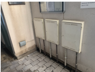
Gas meter cupboards
