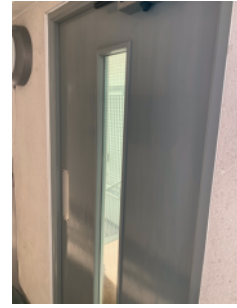
Georgian Wired glazing on staircase
