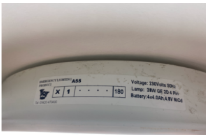
Non-maintained emergency lighting luminaire.
