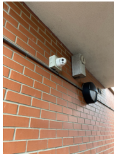
CCTV is installed externally.
