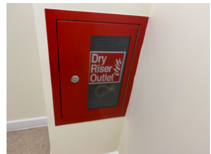
A dry rising main is provided.
