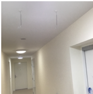
Missing fire escape sign
