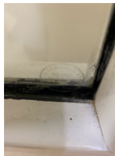
Acid etching visible on staircase door glazing.
