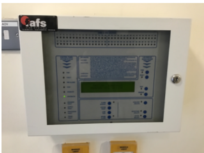
Fire detection panel
