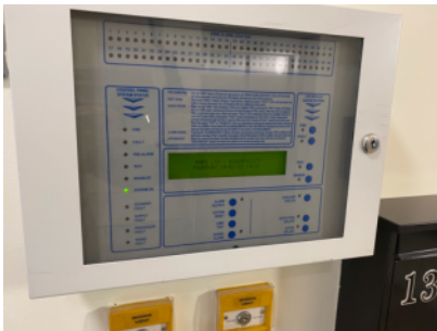
Fire detection control panel with manual smoke vent actuators.
