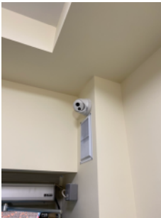
CCTV covering the main entrance.
