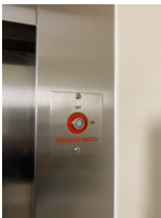
Fireman switch for the control of the firefighting lift.
