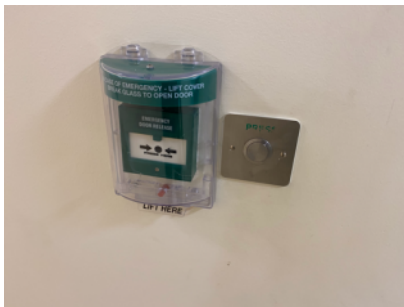
Electromagnetic door release & emergency door release at main entrance door
