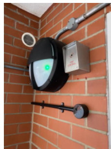
External non-maintained emergency lighting luminaire.
