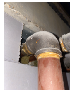
Pipe penetration without adequate fire stopping within riser cupboards.
