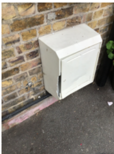
Broken gas meter cabinet.
