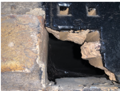
Broken grill above intake cupboard door.
