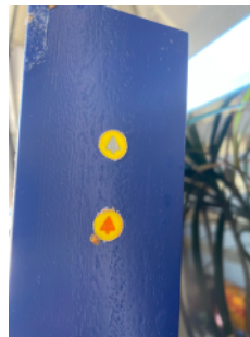
BWF Fire door identification plugs on the new door sets being installed
