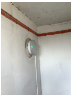
Maintained EL in the staircase
