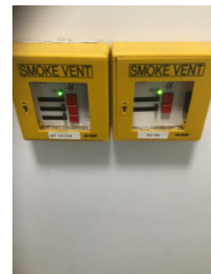
Smoke vent controls - ground floor.
