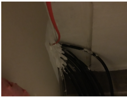
Example of fire stopping within riser cupboards
