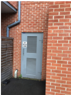
Gas meter room outside the building, not in the common parts.
