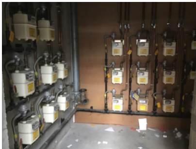
Gas meters located in externally accessed ventilated room.
