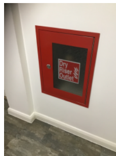
Dry rising main outlet
