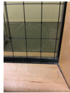
Acid etching on door glazing.
