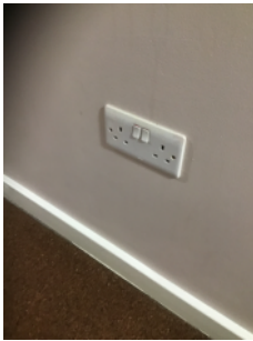
Electrical sockets provided in common areas
