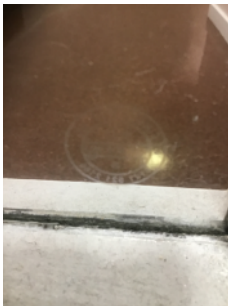
“Pyroguard” FR Glazing in corridor doors.
