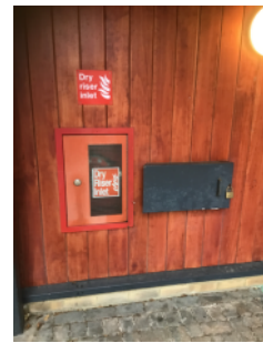
Dry riser inlet
