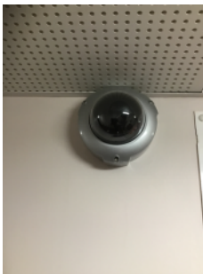
CCTV is provided internally and externally
