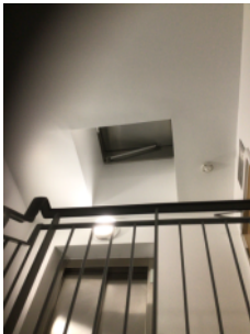
AOV Provided in the staircase
