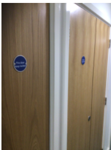
“Fire door keep locked” signage on riser cupboard doors
