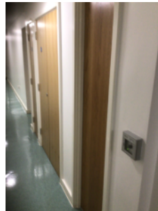
Smoke Shaft door in corridors
