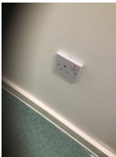
Electrical sockets in common areas.
