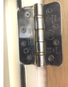
CE1121 Door hinges in riser doors.
