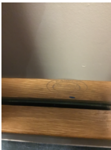
Acid etching on door glazing
