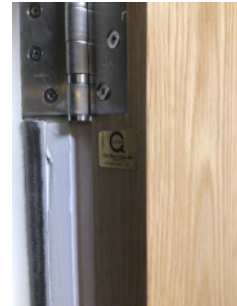
Fire door certifying on riser cupboard doors
