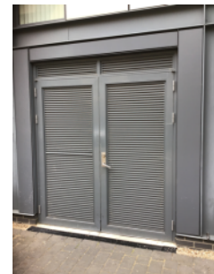
It was not possible to access this external door.
