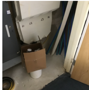
Combustible materials in riser cupboards
