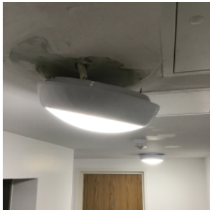
Damaged light fitting on the first floor
