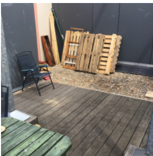
Combustible storage on roof top garden.
