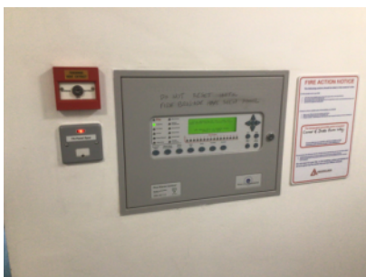
Panel condition at time of inspection.
