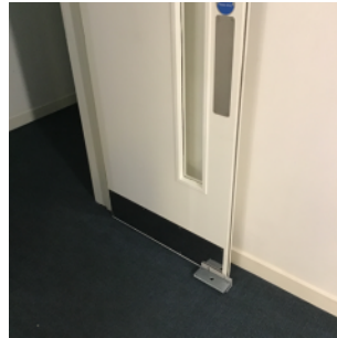
First floor staircase door wedged open
