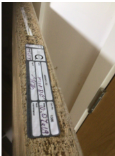
Fire door Certification on riser cupboard doors
