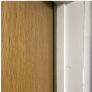
Ground floor corridor door not closing fully
