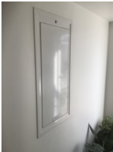
Smoke shaft door in the corridor
