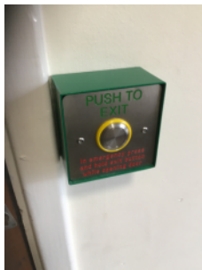
Entrance door override
