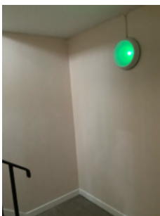
Maintained EL is provided in the escape routes
