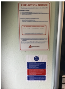
Fire Action Notices - suitable for the stay put policy in place
