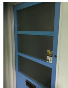
Georgian wired vision panels fitted in FEDs
