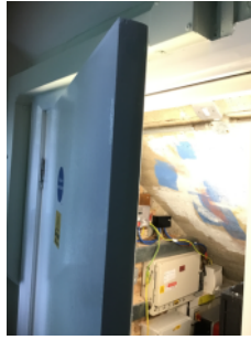
Electrical cupboard door, to FD30S standard.
