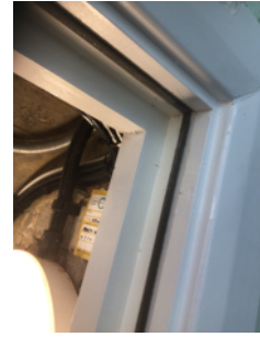
Intumescent strips & smoke seals fitted in electrical cupboard doorframe
