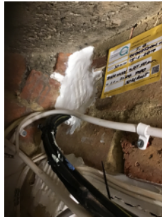
Fire stopping with certification label in electrical cupboard.
