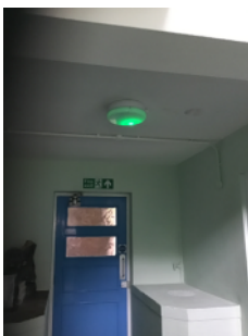
Emergency lighting provided on all levels in the staircase
