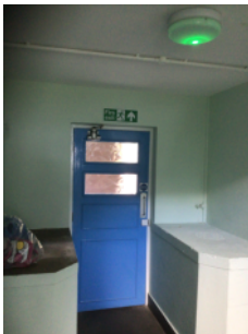
Fire exit sign over rear door.
