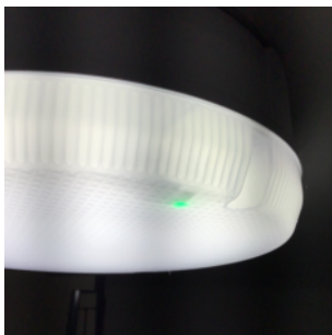
Emergency lighting in staircase
