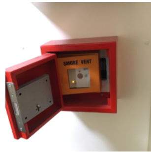
Smoke vent control showing a fault light
