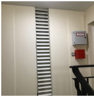
Manual smoke vent and control
