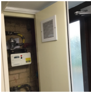
Gas meter cupboard
