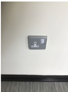
Electrical sockets provided in common staircase
