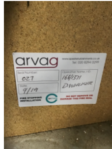
Fire stopping certification label in meter cupboards
