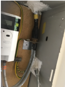
Fire stopping within meter cupboards
