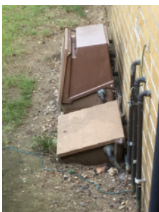
Gas meters located externally
