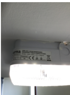
Maintained emergency light units provided in the staircase
