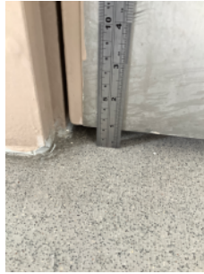
Threshold gap, 20mm, second floor lobby door
