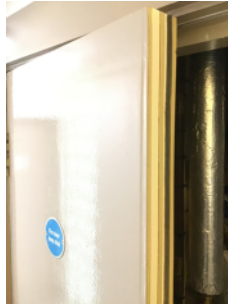
FD60S doors installed in risers.
