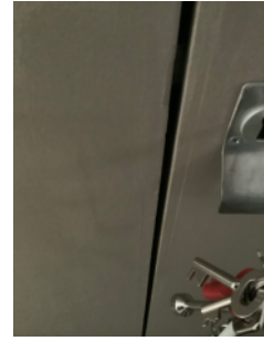
Excessive centre gap on riser door
