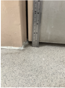
Threshold gap, 20mm, first floor lobby door
