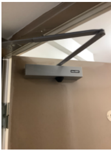
Overhead self closing device on flat entrance doors
