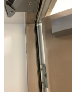
Intumescent strips and cold smoke seals on flat entrance doors
