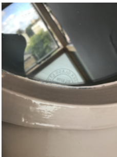
Acid etching on lobby door glazing
