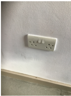
Electrical sockets in common parts
