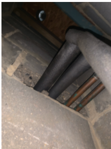
Example of pipe penetrations with no fire stopping in riser cupboards.
