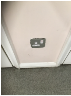
Electrical sockets provided in common areas.
