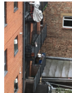
Combustibles being stored on some balconies
