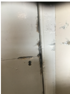
Severe damage to gas meter cupboard door.
