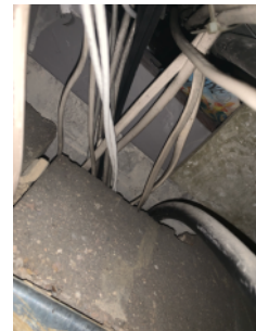
Example of cable penetrations with no fire stopping in riser cupboards.
