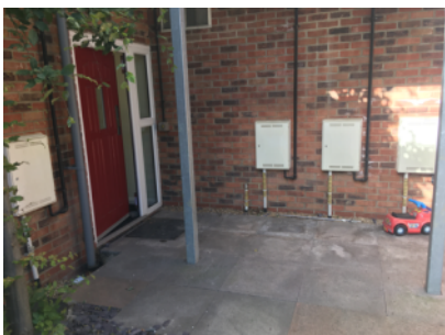
Gas meters located externally
