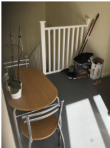
Obstructions in escape routes
