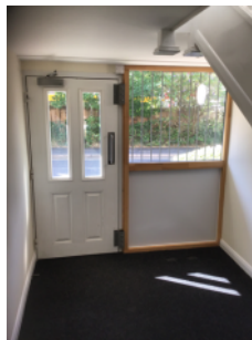
No fire exit sign over main entrance door to street
