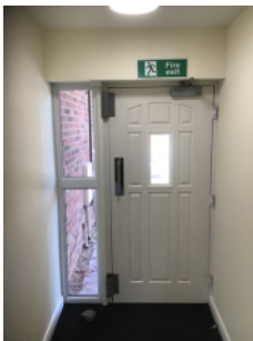
Fire exit sign over rear door to courtyard
