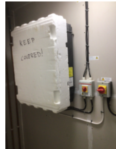
Photovoltaic controls in riser cupboard on 2nd Floor
