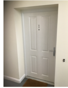
Example of flat entrance doors installed in the building
