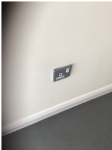
Electrical sockets provided in common areas
