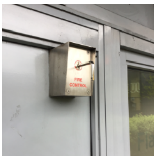
Defective override control
