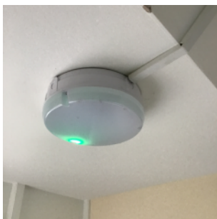
Emergency lighting in staircase
