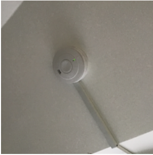
Part 6 smoke alarm in staircase
