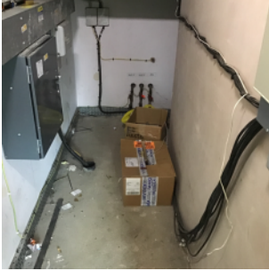
Discarded cardboard in electrical cupboard
