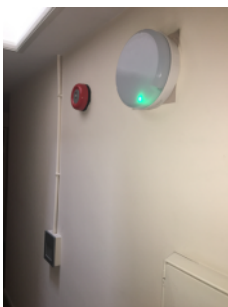
Maintained (local) emergency lighting provided in the common parts
