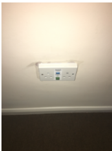
Electrical sockets provided in common area
