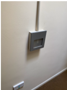
Break-glass manually operated ventilation system
