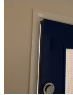
Automatic self-closing cross-corridor door not closing fully
