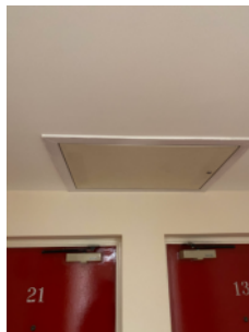
The roof space was not inspected within the scope of this FRA
