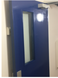
Automatic self-closing corridor doors - tested during inspection
