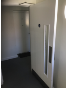
Automatic FD30S SC doors provided on the staircase
