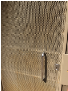
Vented door to gas meter cupboard
