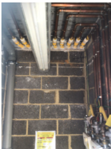
Fire stopping within the gas meter cupboard
