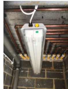
Intrinsically safe strip light within the gas meter cupboard
