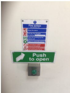
Incorrect fire action notice.
