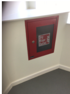
Dry riser outlets provided within the staircase
