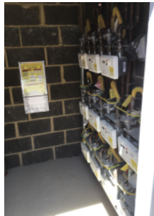
Gas installations in external gas cupboard/room.
