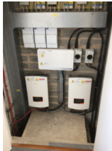
Photovoltaic generator isolator in third floor riser
