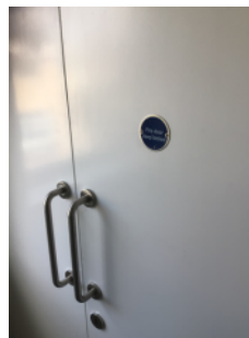
Fire Door Keep locked signage on riser doors
