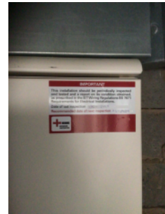
Evidence of fixed electrical installation inspection in May 2019
