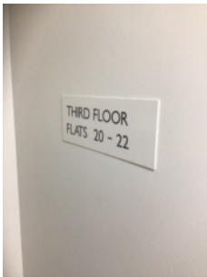
Floor numbers are clearly identified
