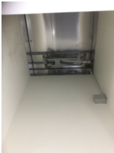
AOV at the head of the staircase
