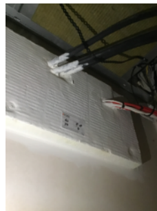
Example of fire stopping installed, with certification label.
