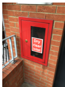
Dry riser inlet, adjacent main entrance door.
