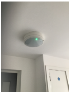
Maintained emergency lighting is provided in the common staircase
