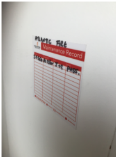
Evidence of dry riser testing
