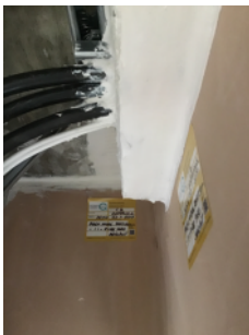
Evidence of Fire Stopping in risers cupboards
