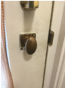
Thumb turn device provided on the main entrance door.
