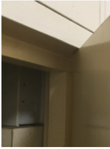
25mm door stops on electrical cupboard.
