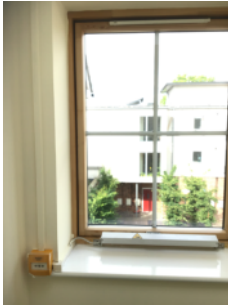
Smoke vent manual actuation with window AOV
