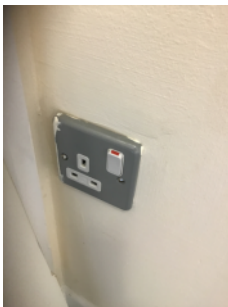
Electrical sockets provided in common areas
