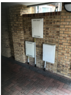
Gas meters located externally
