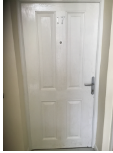
Example of flat entrance doors installed in the building
