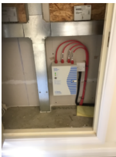
Main Smoke vent control
