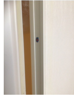
BWF Certifire plug in hinge edge of No 15 flat entrance door
